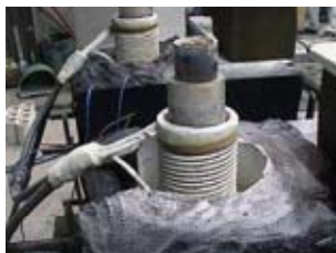
Casting process using Induction heating riser system Developed jointly by Tajima Light Metals Co., Ltd., Daihatsu Metal Co., Ltd., and Dai-ichi High Frequency Co., Ltd.
