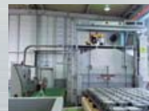
Large-scale heat treatment furnace
